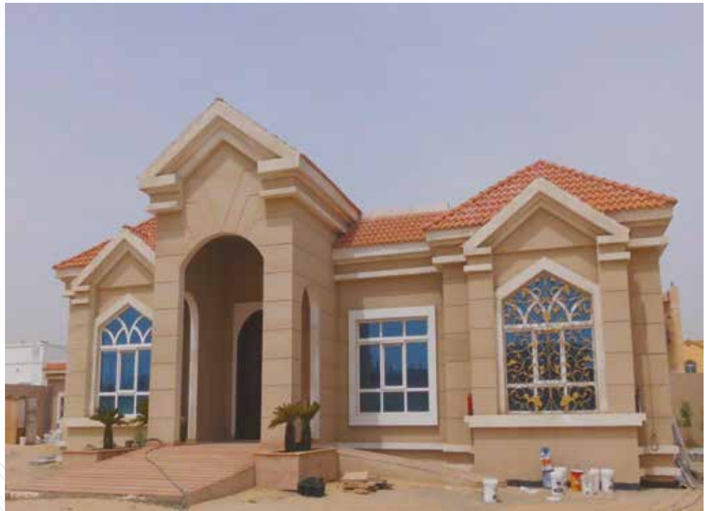
G+1 VILLA, KHAWANEEJ CONSULTANT: M/S ADNAN SAFFARINI CONTRACTOR: M/S MIAMI CONTRACTING LLC CLIENT: MR.KHATER HASSAN ALI KHAMIS BIN KATER
